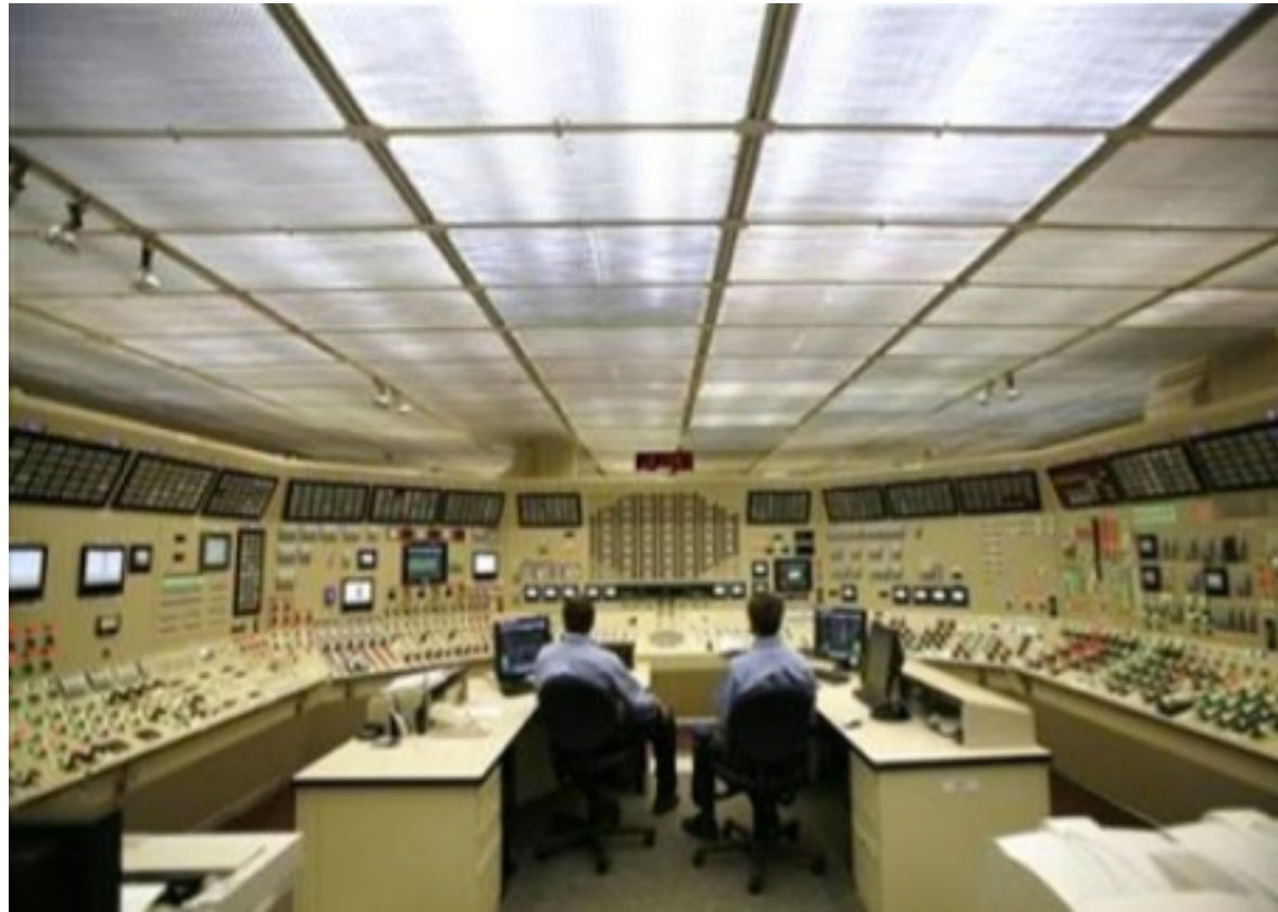
Power plant control room
